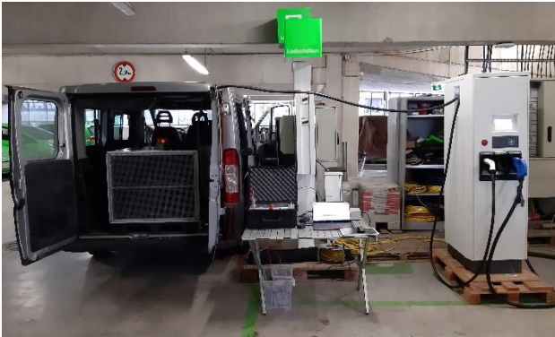
Figure 2: Test setup consisting of the demonstrator (left), the control unit (centre) and the DC charging station to be tested (right).
